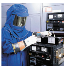
Exhibit 110.7 Electrical worker clothed in personal protective equipment (PPE) appropriate for the hazard involved. 2
